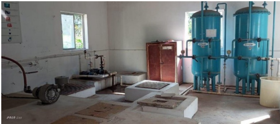
Pic: Sewage water treatment plant
