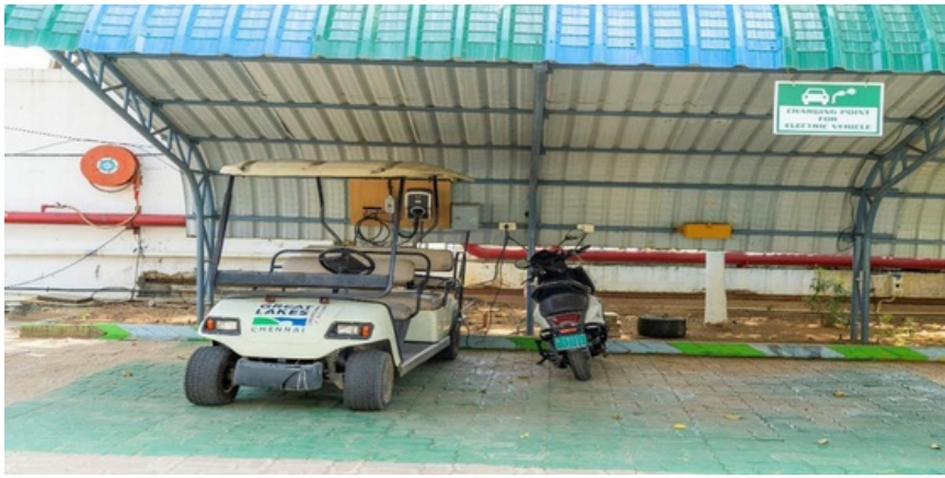
Pic: EV charging station
