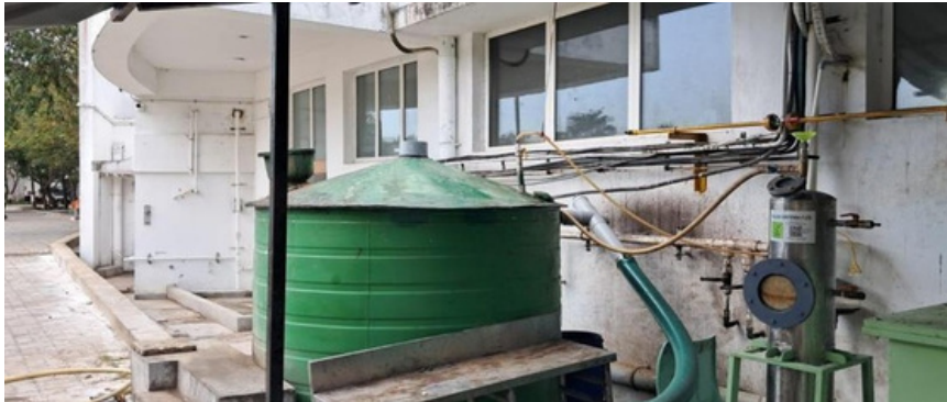
Pic:Bio Gas Plant
