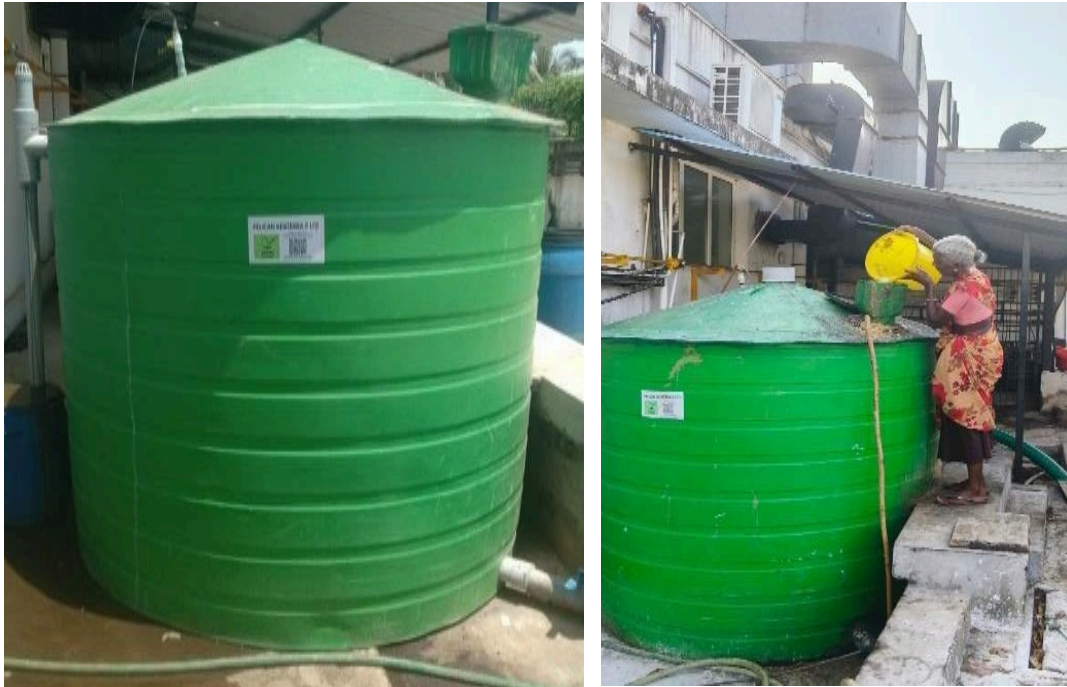
Pic: Bio gas plant
